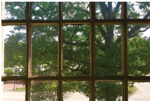
The windows in Friends Hospital still have the original iron sashes and mullions, which were painted to look like wood and not prison bars.
